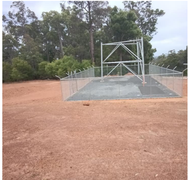
Photo 2 Telecoms tower and fencing
