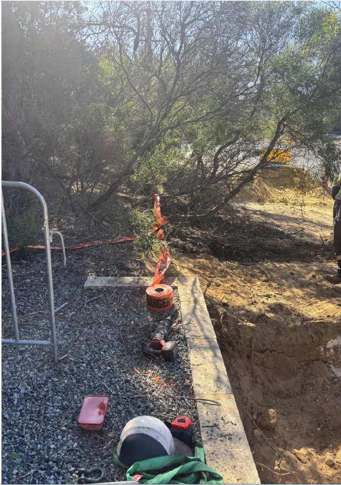
Image 8: Additional 12.5m x 1.5m clearing area to facilitate cable connection to RMU.
