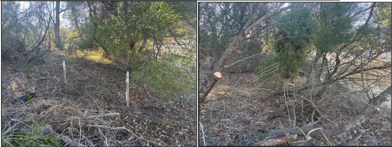
Image 9 & 10: Additional 12.5m x 1.5m clearing area to facilitate cable connection to RMU.
