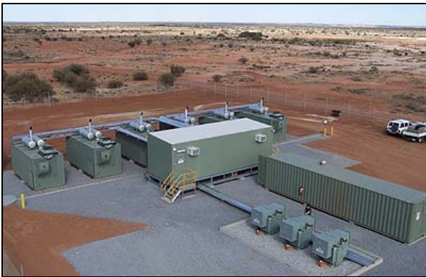
Above - The new Yalgoo Power Plant, 2006.
