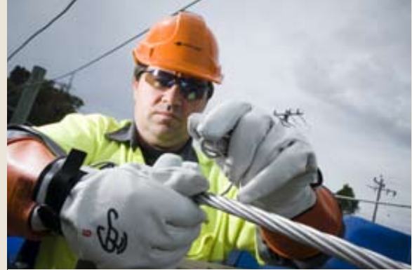
Training and Development Officer Dave Matthews demonstrates the correct use of gloves in a low voltage environment.
