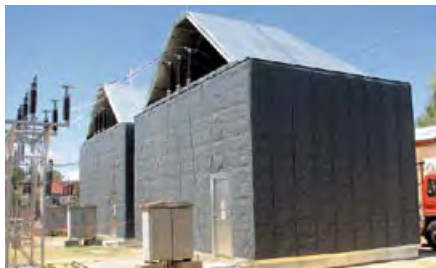
Putting 'curtains' around substations is reducing noise impact in the community.
