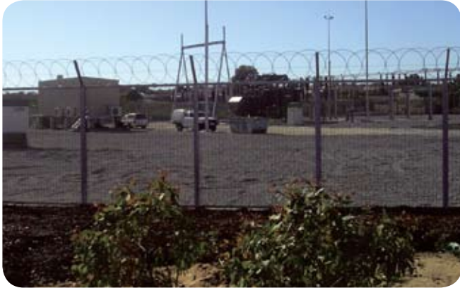
An example of substation fencing
