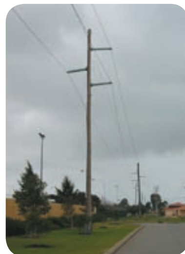
Example of 132 kV timber pole
