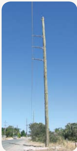
132 kV wood pole configured as a running post with overhead earth wire.
