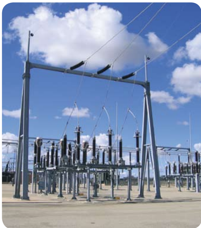
Transmission voltage connection at Merredin Terminal.
